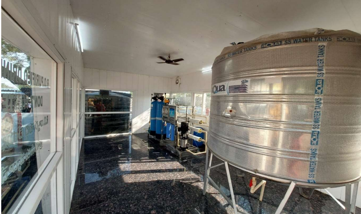
Pic 25 – Inside view of the RO plant
