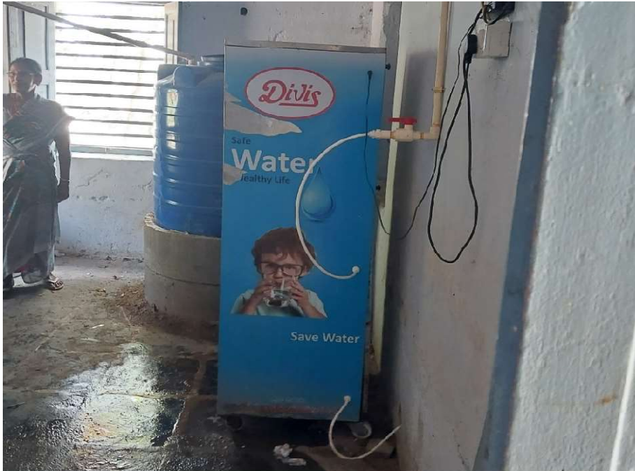
Pic 9 – RO water purifier kept in a separate room under the supervision of Aaya
