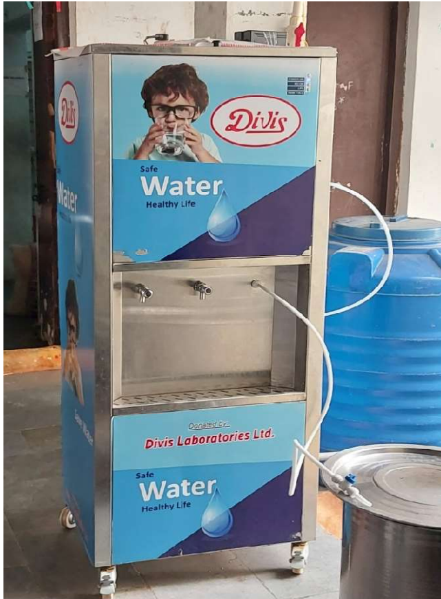
Pic 6 - Unit with facility to fill water drum
